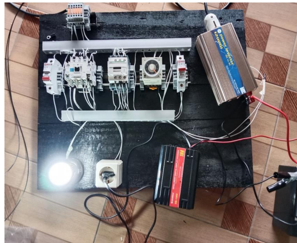
Figure 4. PLN in OFF Conditions
