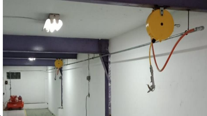
Figure 3. The Result of the Design Of The Wind Pipe Installation Using A Solenoid Valve
